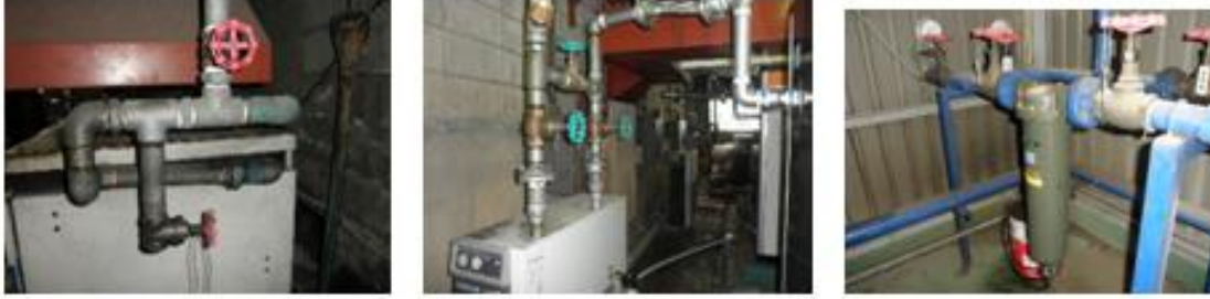
Example of pipes having many valves or bends, generate resistance and pressure loss. Change the type of the valves (to the one with low resistance) or reduce bends as much as possible.
