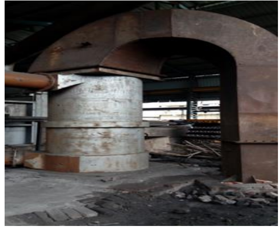
Waste heat recovery system
