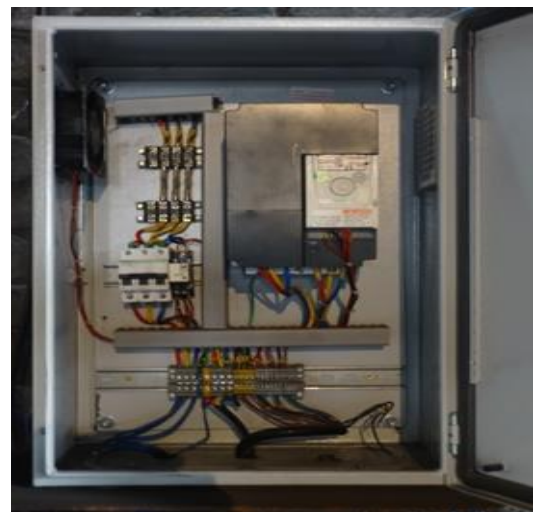
VFDs to regulate combustion air
