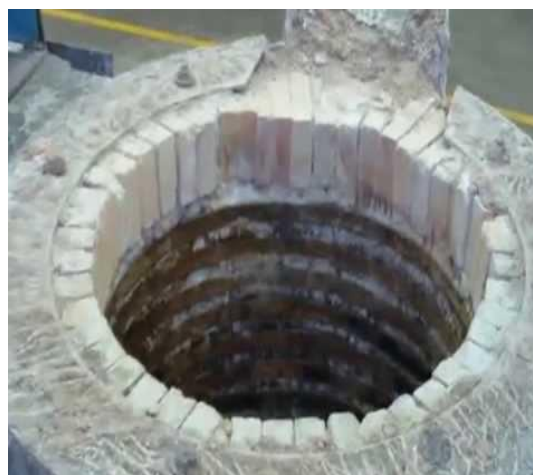
Figure 2.5: Induction furnace working lining
