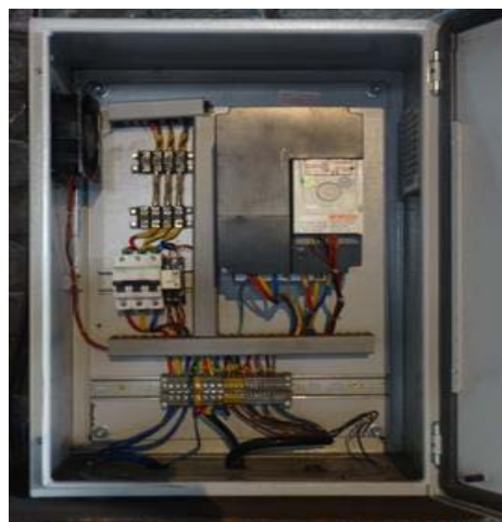
Figure 5.4: VFDs to regulate combustion air
