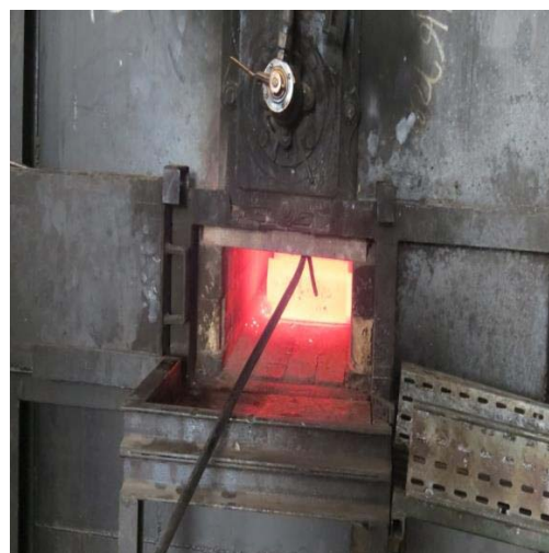
Figure 5.3: Re-heating furnace discharge door
