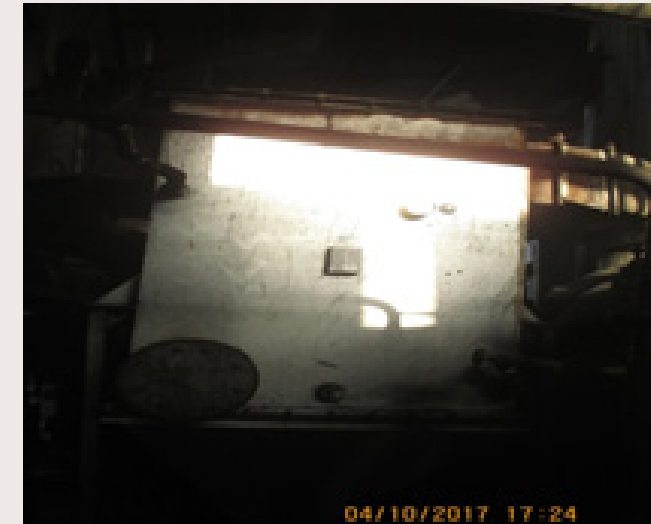
Thermic fluid exist with economizer at Simandhar Fabtex
