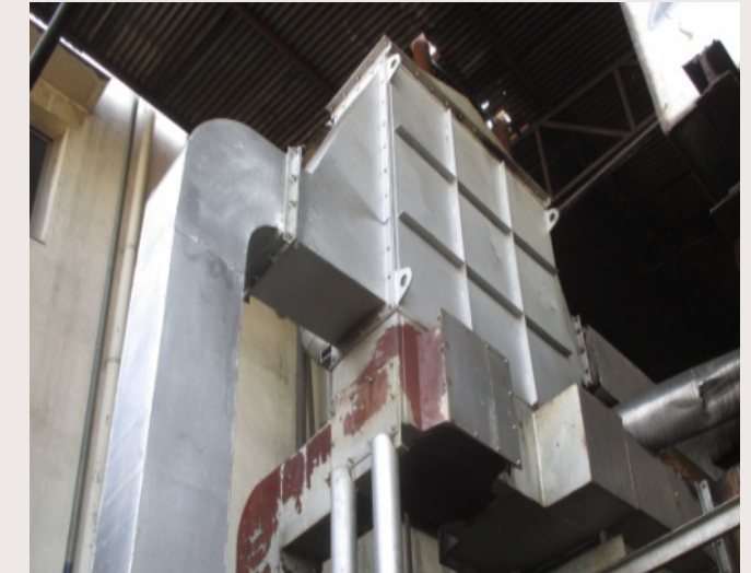
Air pre heater installed at Simandhar Fabtex
