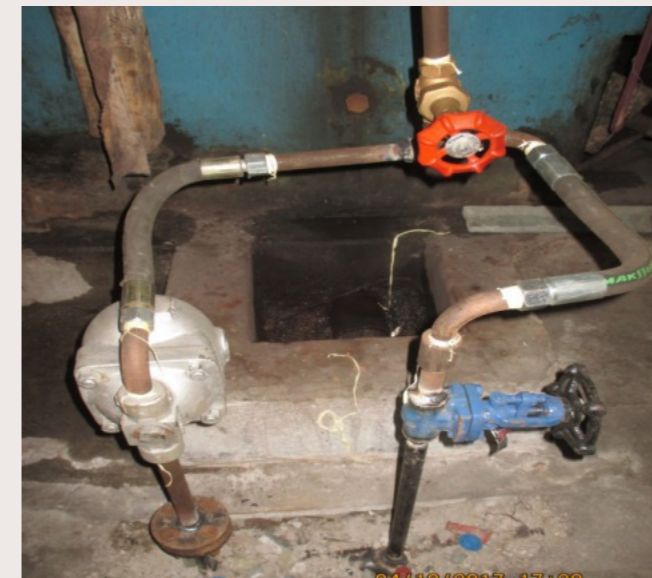
Float trap installed at Simandhar Fabtex
