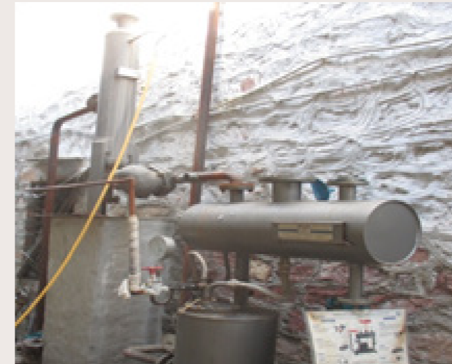
Jet dyeing with condensate recovery system at Manoj Dyeing
