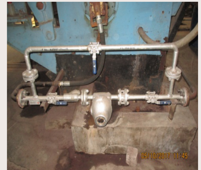
Float trap installed at Rajaram Mills
