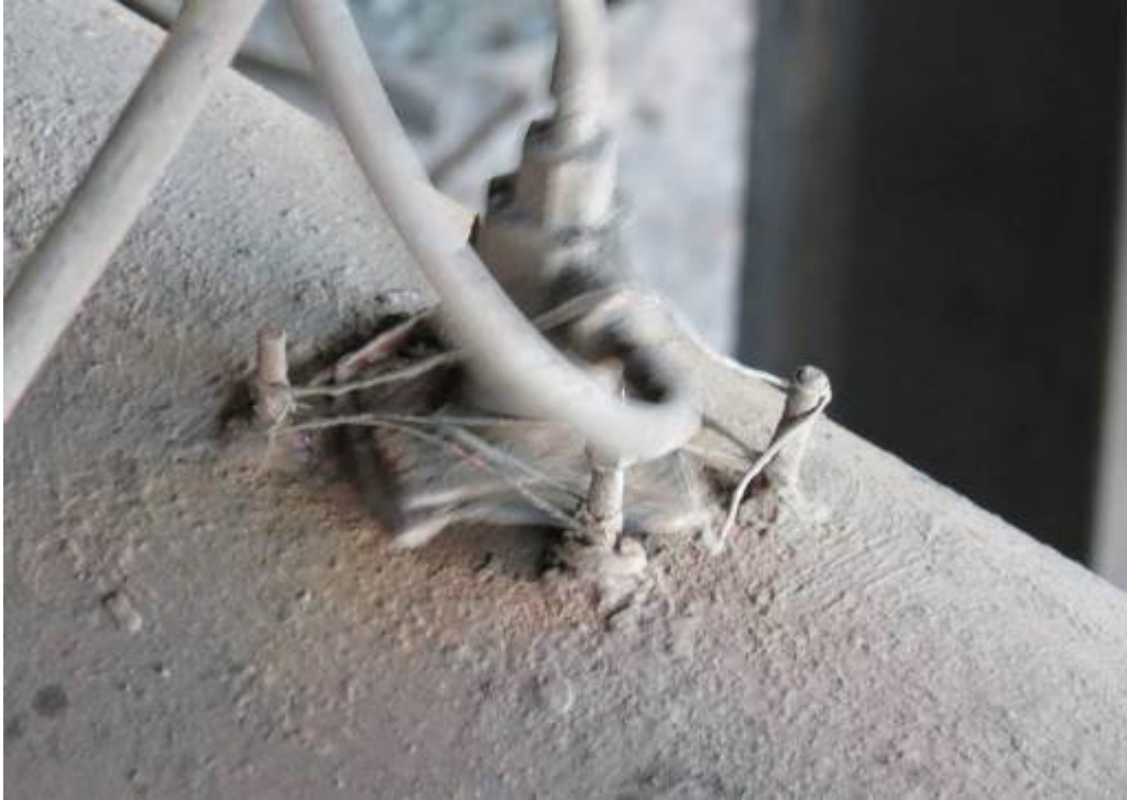
Figure 2.17: Pressure measurement point on the air supply line
