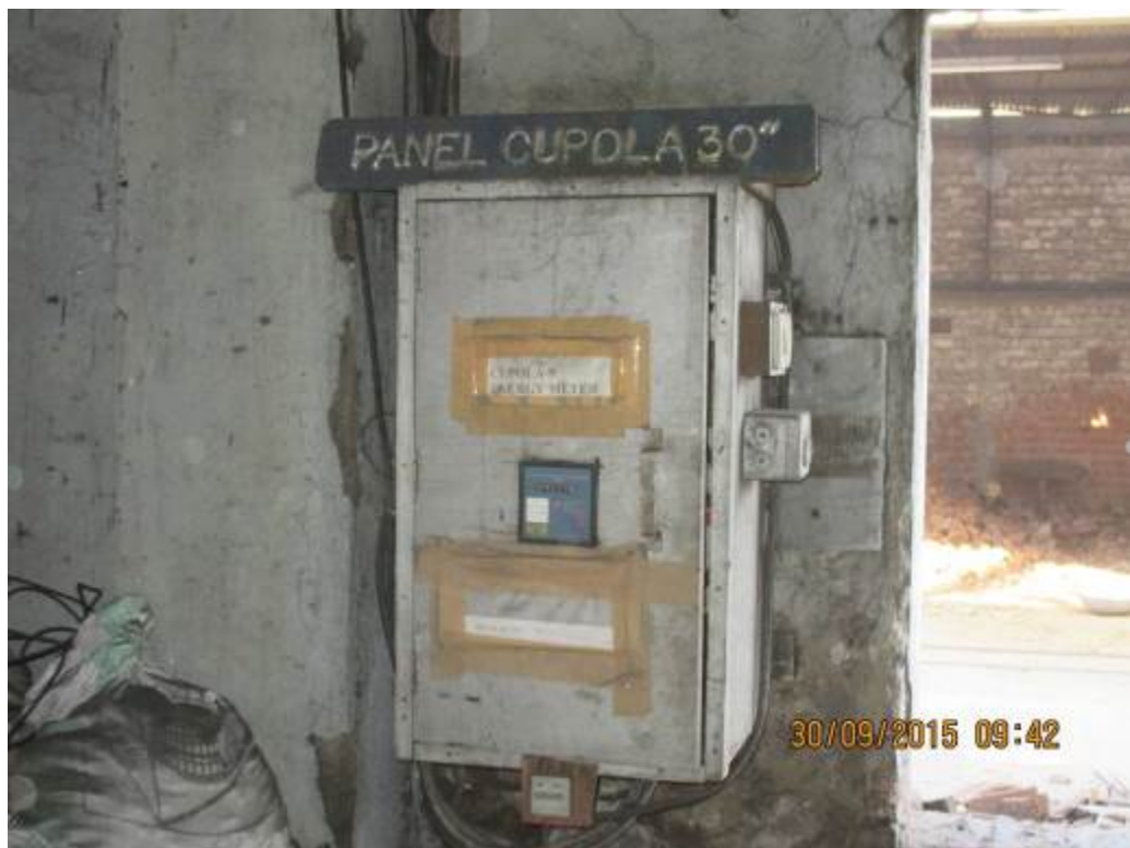
Figure 2.20: Cupola power supply panel
