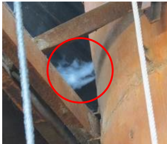
Figure 2.26: Leakage on cupola wall
