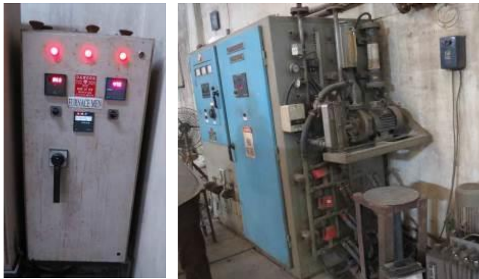
Figure 2.26: Separate panel for electricity supply to induction furnace, Electrical panel of induction furnace
