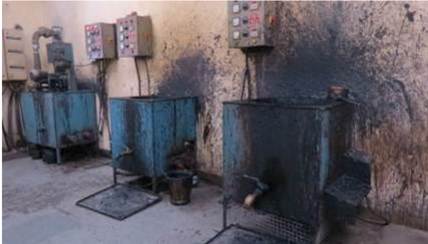
Figure 2.2: Wax melting in thermic oil heaters
