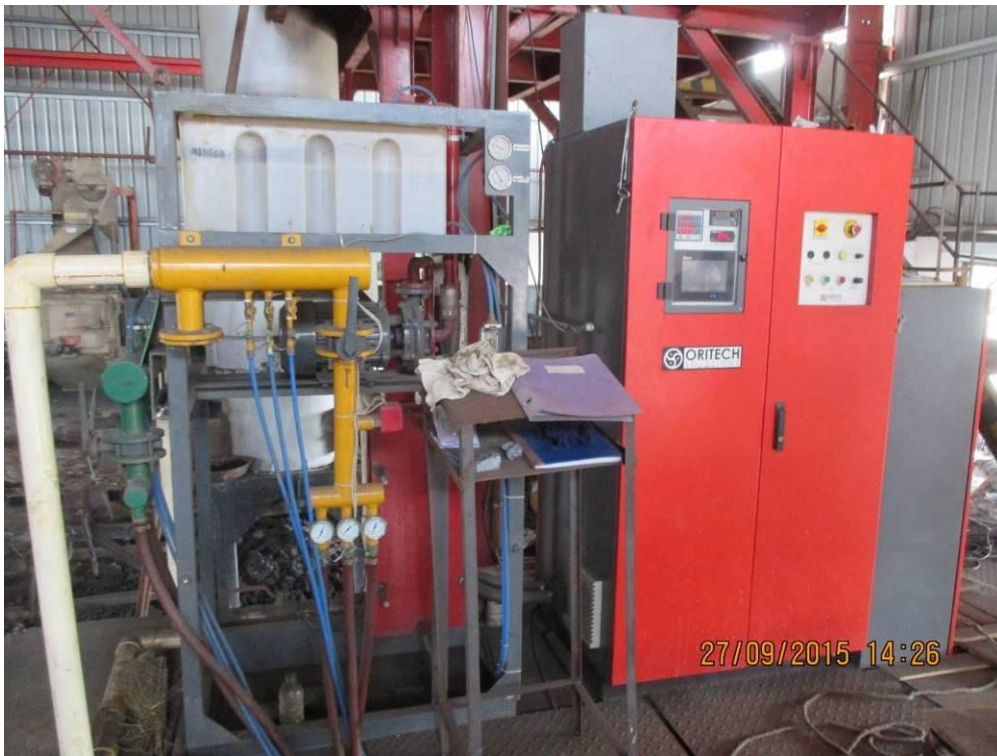
Figure 2.5: Induction furnace control panel
