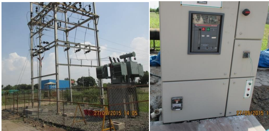
Figure 2.19: Pictorial depiction of transformers and electrical panel installed
