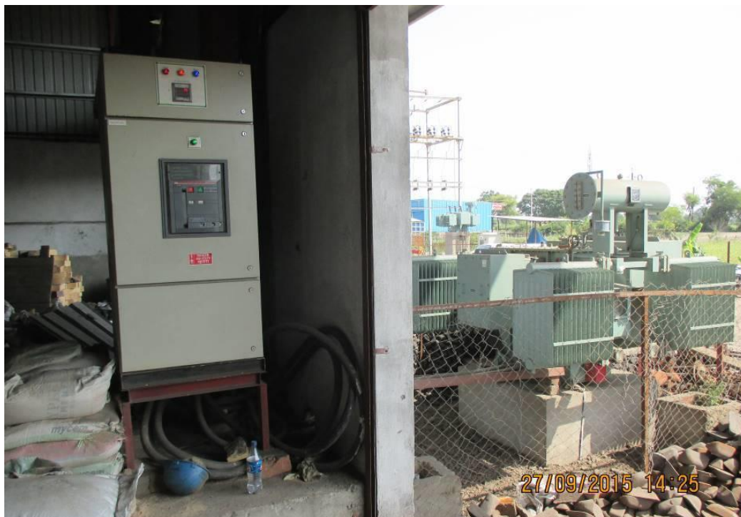
Figure 2.21: Separate panel for electricity supply to induction furnace, Electrical panel of induction furnace
