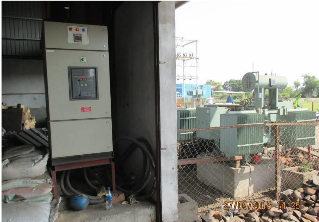
Figure 2.6: Separate transformer and energy meter for induction furnace
