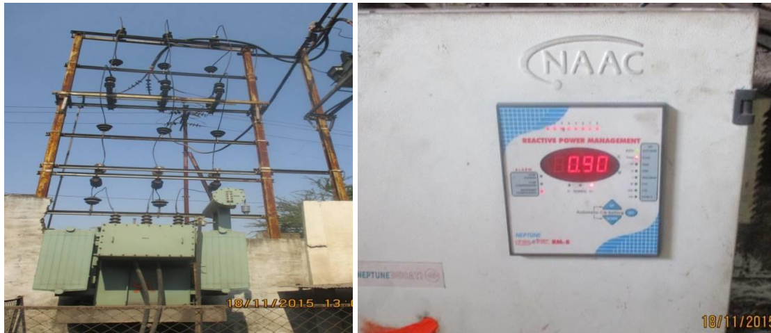
Figure 2.22: Pictorial depiction of transformers and APFC Panel installed
