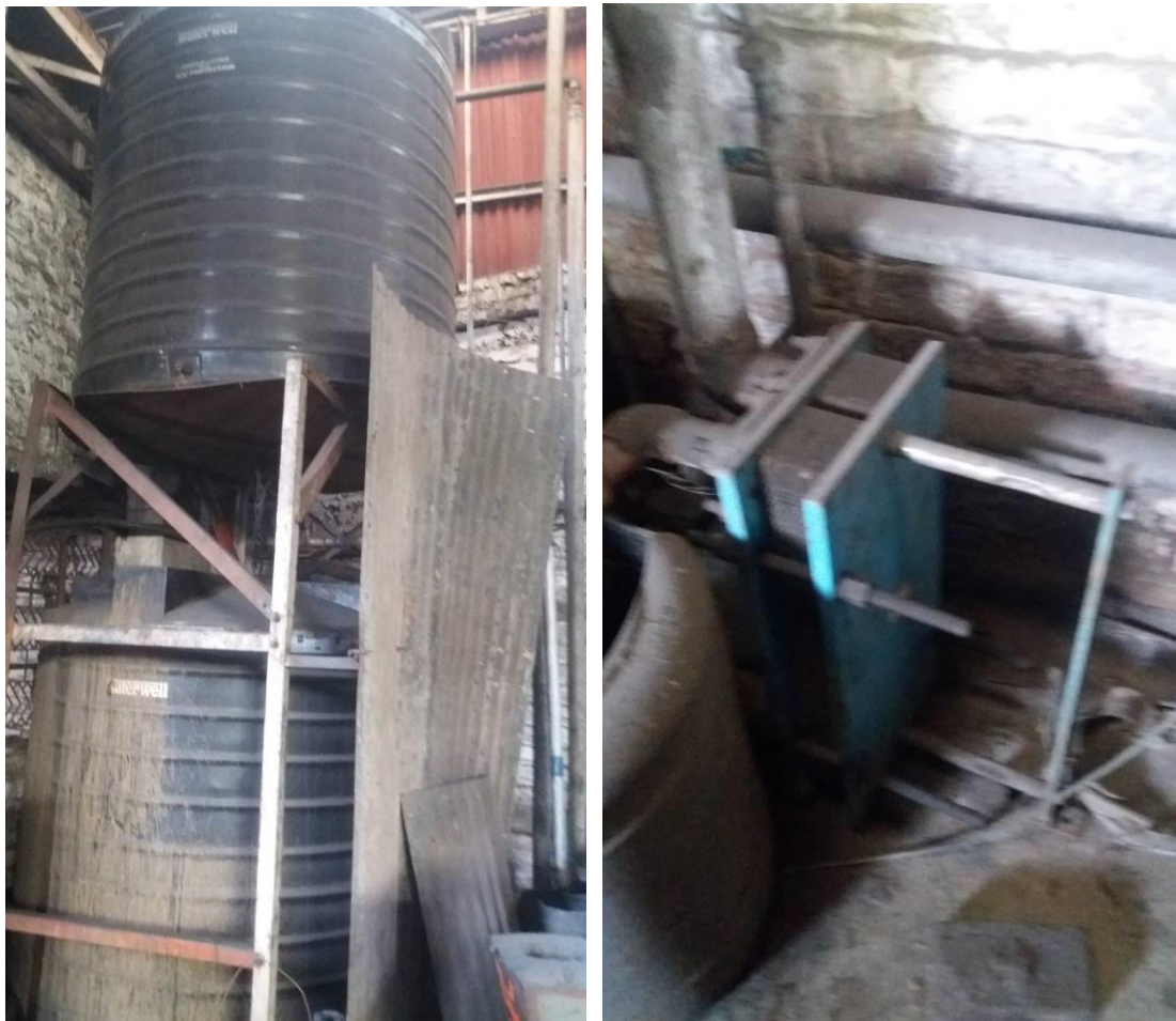
Figure 2.11: Raw water and soft water storage tank and heat exchanger being used in the cooling circuit
