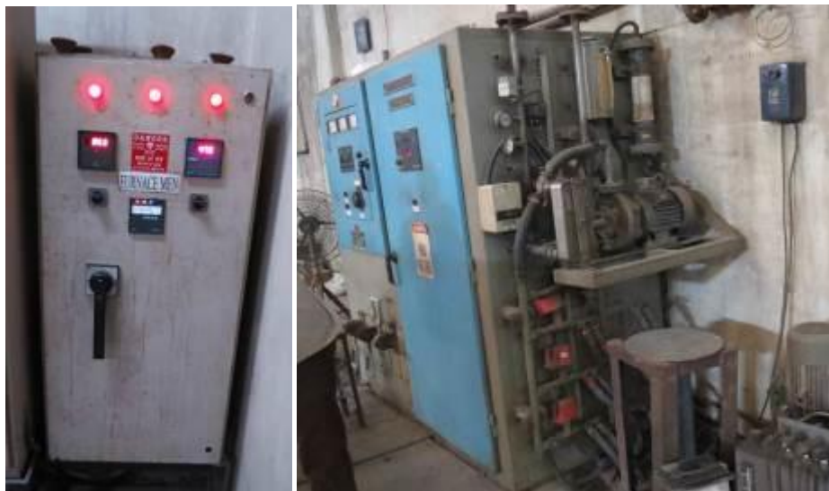
Figure 2.21: Separate panel for electricity supply to induction furnace, Electrical panel of induction furnace
