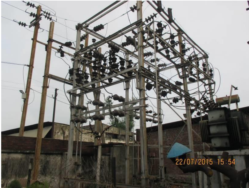
Figure 2.20 (a): Pictorial depiction of transformers installed
