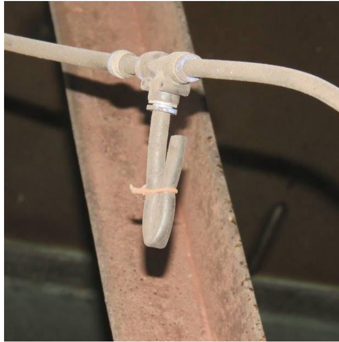
Figure 2.25: Temporary arrangement made to prevent air leakages
