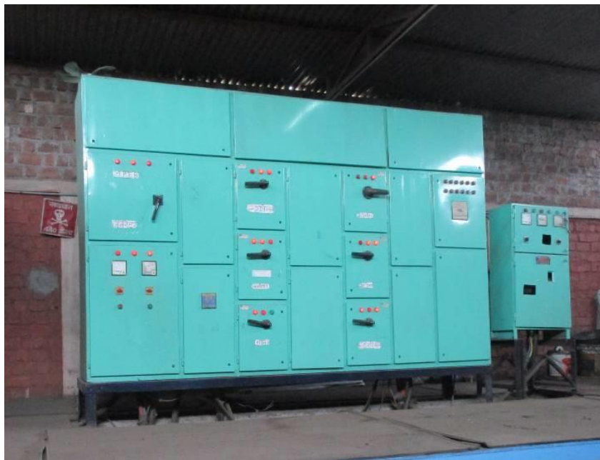
Figure 2.20 (b): Pictorial depiction of electrical panels installed
