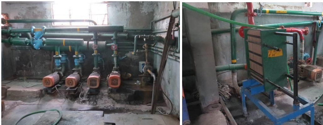
Figure 2.24: Pumps and plate type heat exchanger being used in cooling circuit
