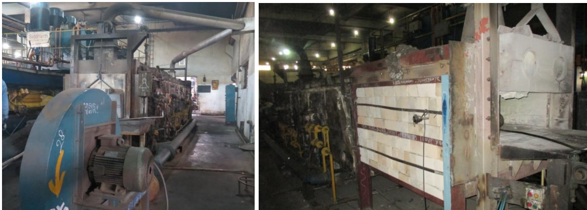
Figure 2.8: Reheating furnace for heating of billet pieces
