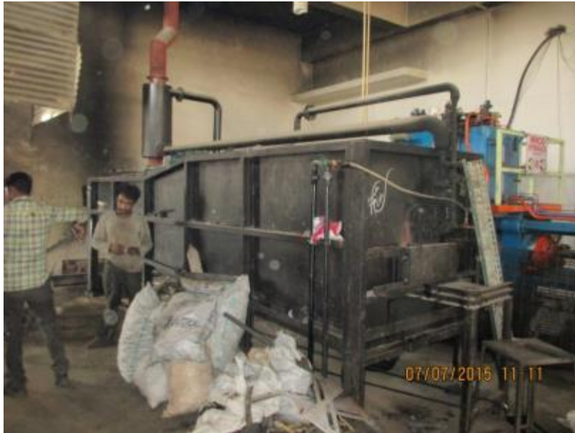
Figure 2.8: Oil fired Reheating furnace
