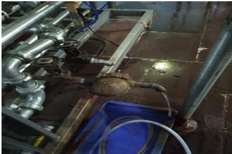
Figure 14: Condensate drained out
