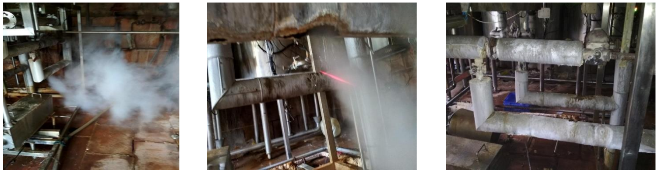
Figure 16: CIP trap bypassed
