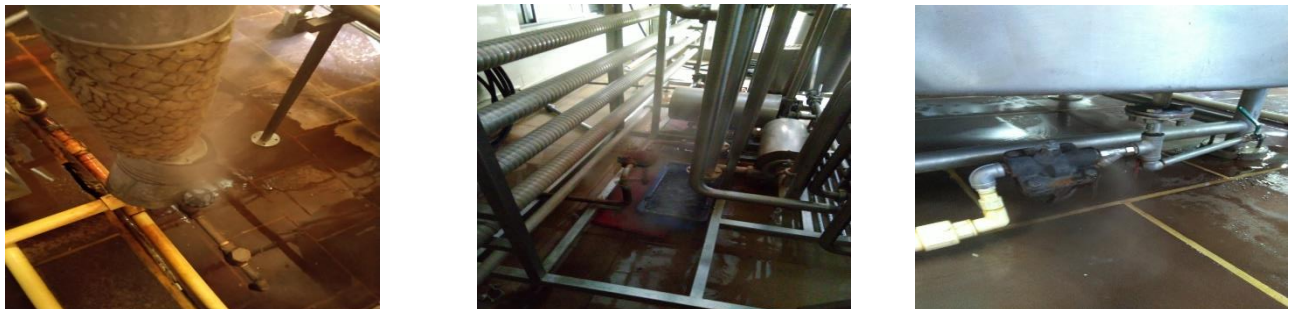
Figure 13: Trap and Steam Leakage
