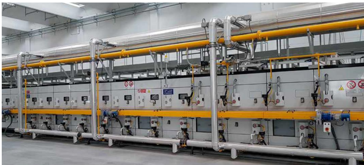
Figure 31: Heat recovery system for combustion air
