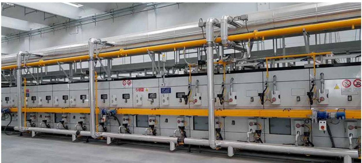
Figure 22 : Heat recovery system for combustion air
