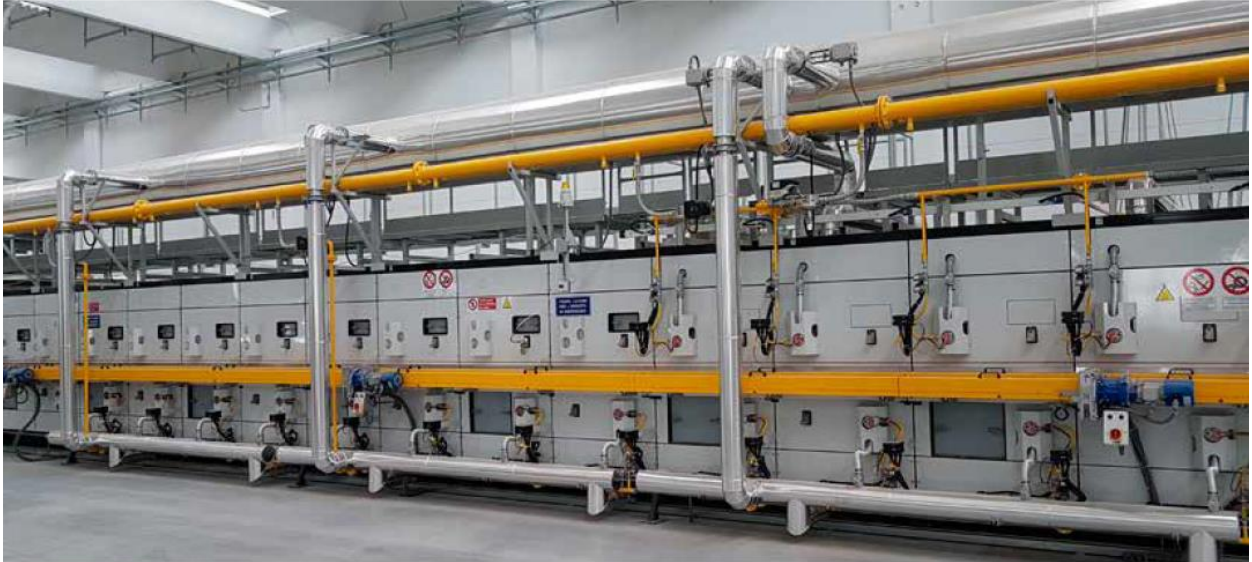
Figure 17 : Heat recovery system for combustion air
