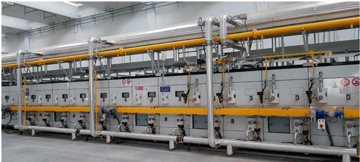
Figure 18 : Heat recovery system for combustion air
