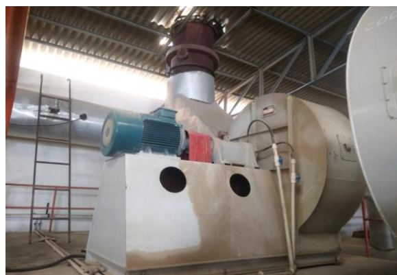
Figure 25: Direct driven blower fans
