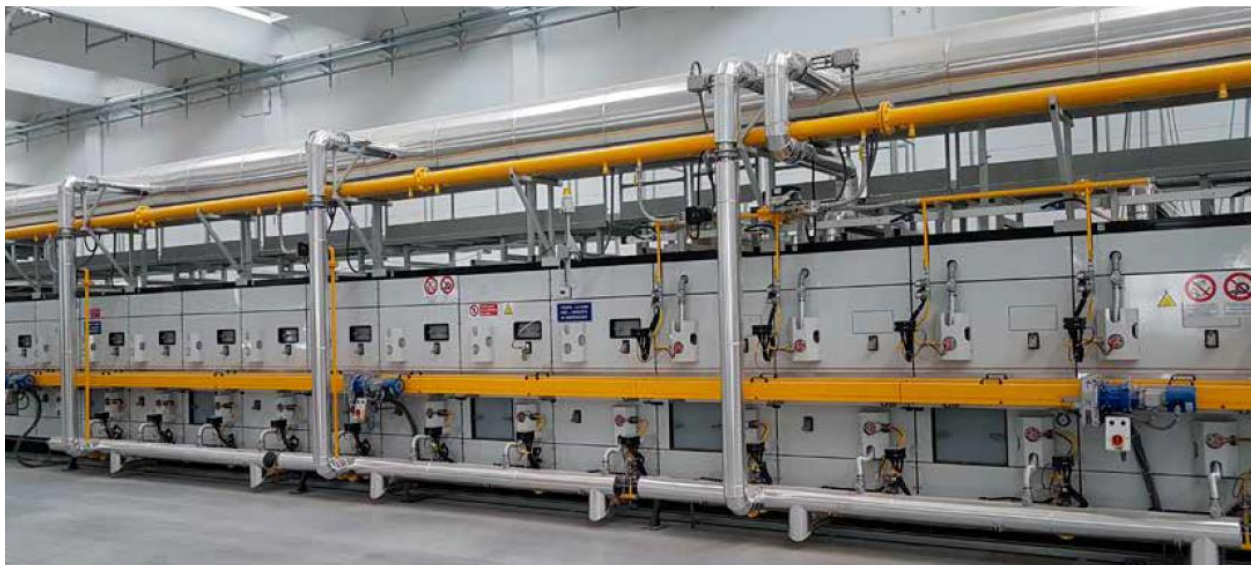
Figure 18 : Heat recovery system for combustion air
