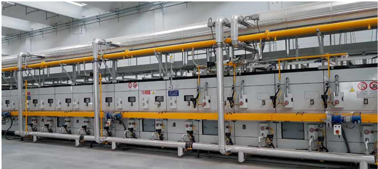
Figure 20 : Heat recovery system for combustion air
