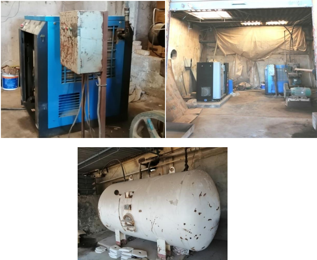
Figure 17: Compressors and receivers
