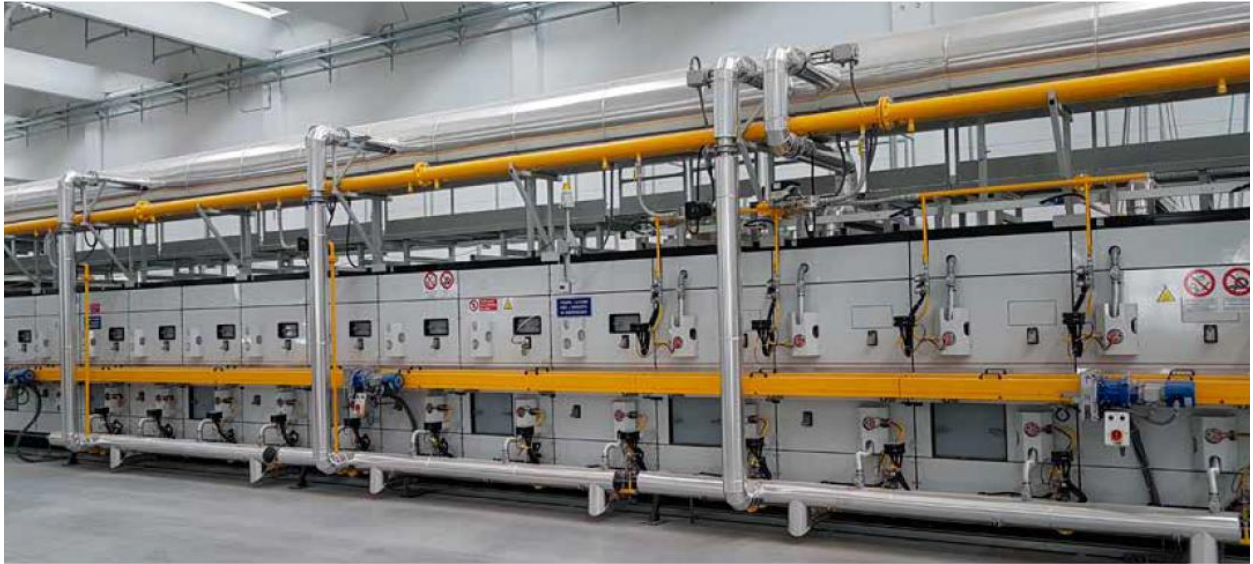
Figure 29: Heat recovery system for combustion air
