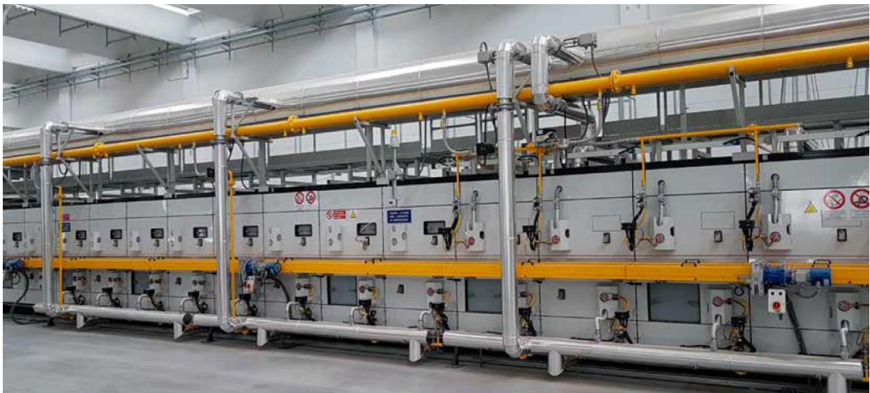
Figure 22: Heat recovery system for combustion air
