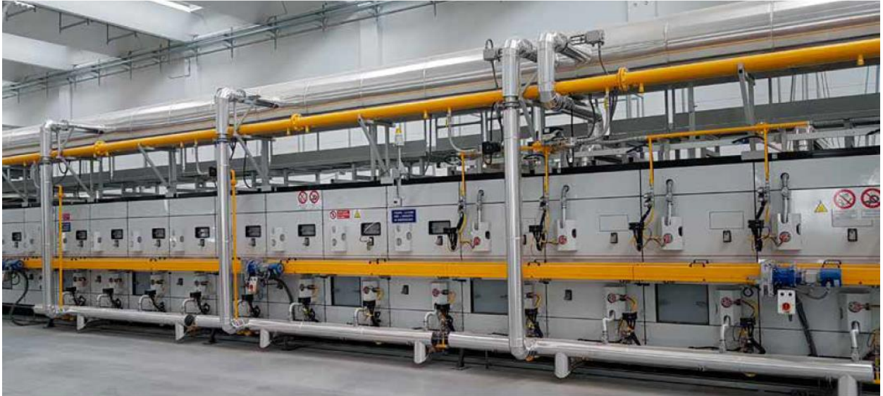
Figure 21 : Heat recovery system for combustion air
