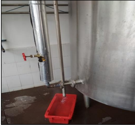
Figure 9: Condensate from CIP
