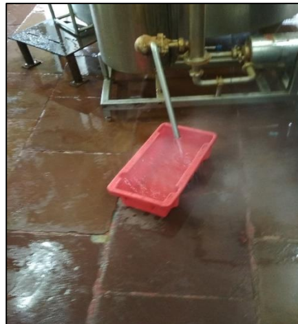
Figure 11: Condensate from hot water tank
