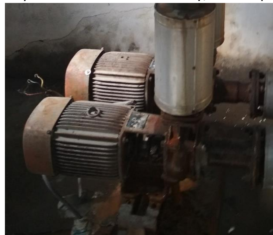
Figure 13: Old Chilled Water Pumps
