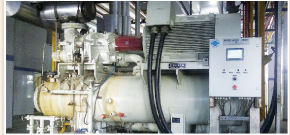
Air compressor at refrigeration plant
