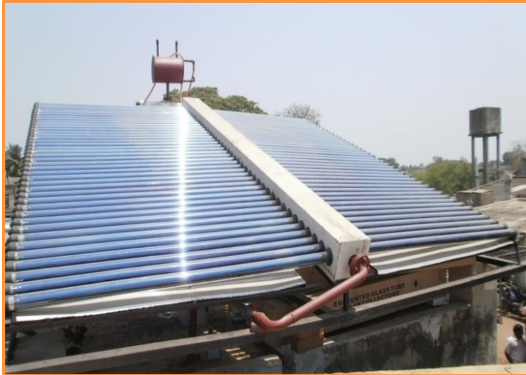
Single Module ETC type Solar Thermal System
