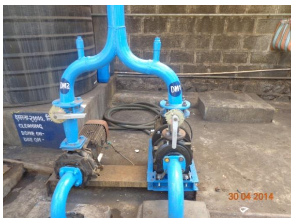
Proper sizing of pump and improving energy efficiency
