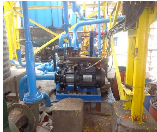
Removal of obstruction to cooling tower air intake and FRP blades
