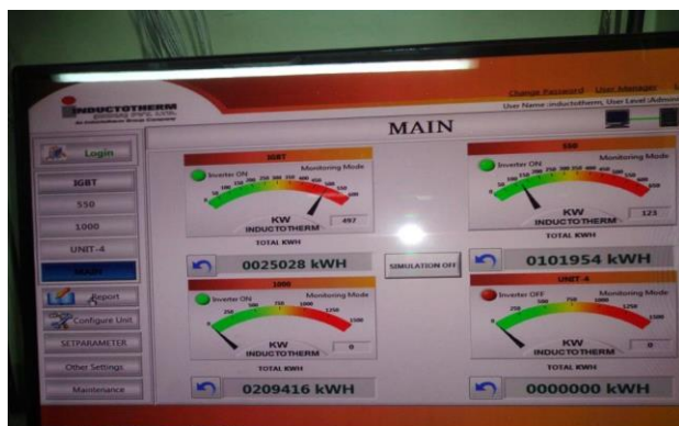
Installation of induction furnace energy monitoring system
