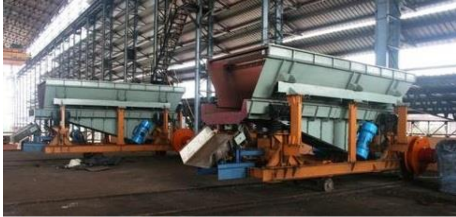
Figure 2.1.4a: Vibrating feeder for induction furnace
