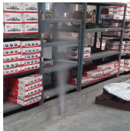
Compressed air leakage
