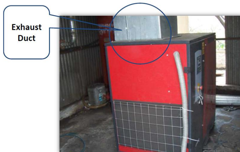
Exhaust duct for air compressor
