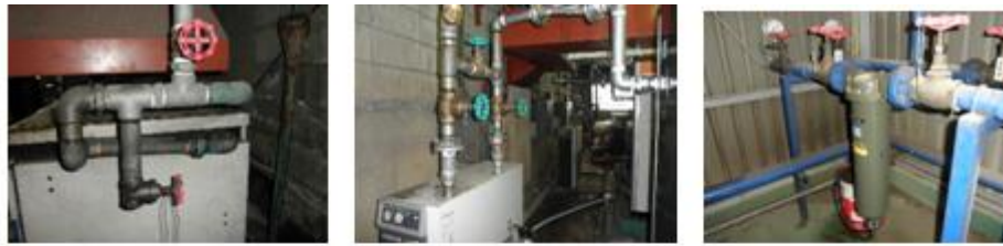
Example of pipes having many valves or bends, generate resistance and pressure loss. Change the type of the valves (to the one with low resistance) or reduce bends as much as possible.
