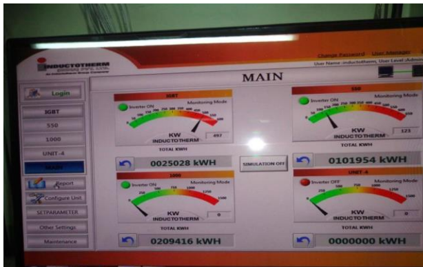
Installation of induction furnace energy monitoring system
