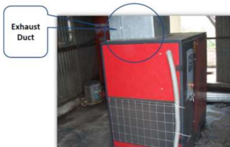
Exhaust duct for air compressor
