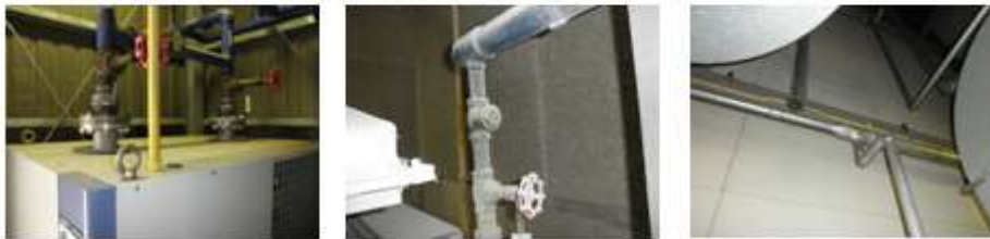
A pipe narrowed immediately after the air dryer. Generates resistance and pressure loss. A riser pipe. Causes a backward flow of condensate, leading to an increasing number of mechanical troubles.
