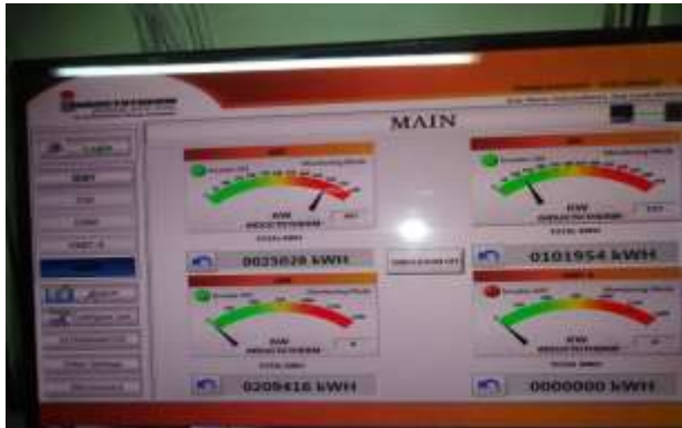
Installation of induction furnace energy monitoring system
