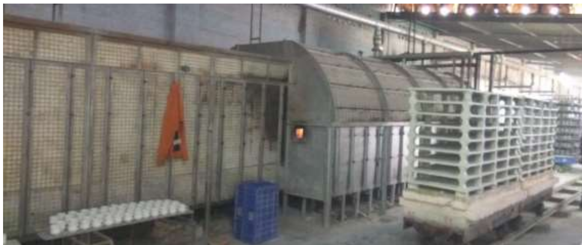
Tunnel kiln in Khurja cluster
